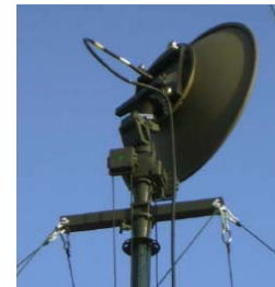
Band 4 antenna mounted on telescopic support mast with rotator/tilter
